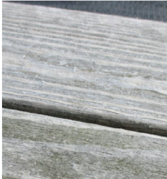
Naturally occurring surface fibres on decking
